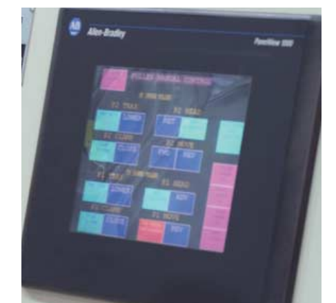
SCSExtrude coordinates the extrusion process, enabling communication among individual machines.
